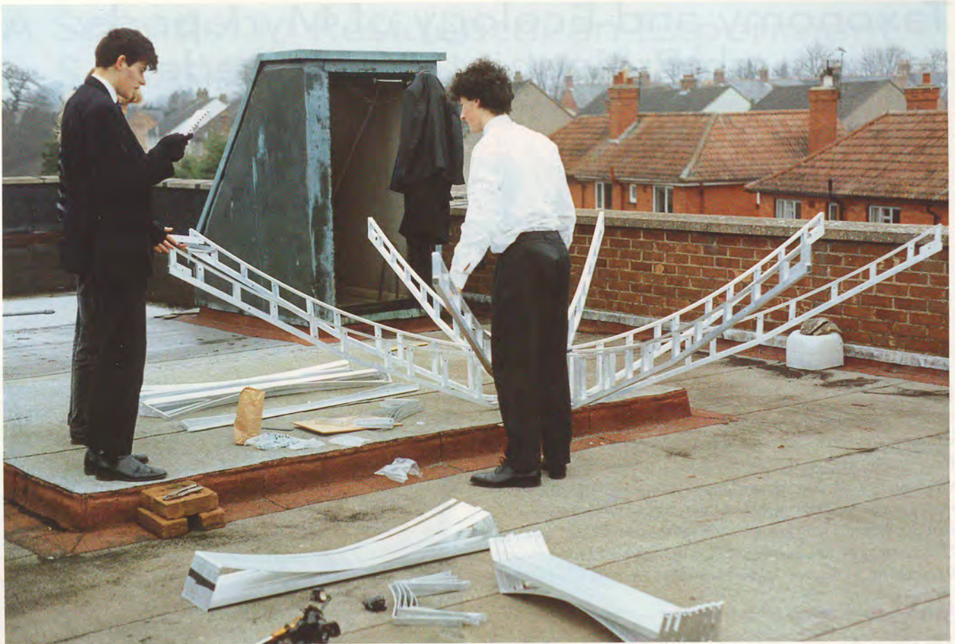
Sixth form students constructing a 4m satellite dish for Radio Astronomy at 1420 MHz.
